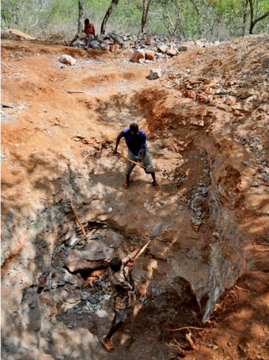
Figure DD-12. Digging a trench at a hard-rock mine. Photo © V. Pardieu/GGL.
