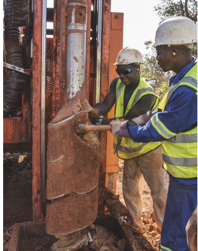
Figure 10. Workers remove the soil and gravel that come up with the auger and then dump the material into a container for further processing. Photo by Andrew Lucas/GIA.
